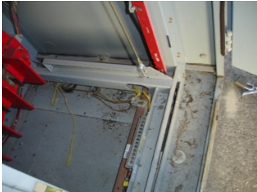
MCC-03 Future 350HP Pump Starter Section Conduit Entry
